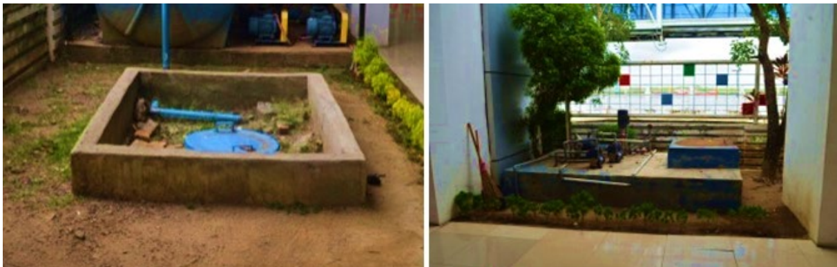
Figure 12 : Ground Water Tank & Septic Tank at Belawan Passenger Terminal Building ( Source : Documentation) Author , 2024)
