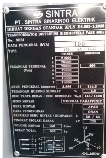
Figure 3. Transformer name plate after Upgrading
