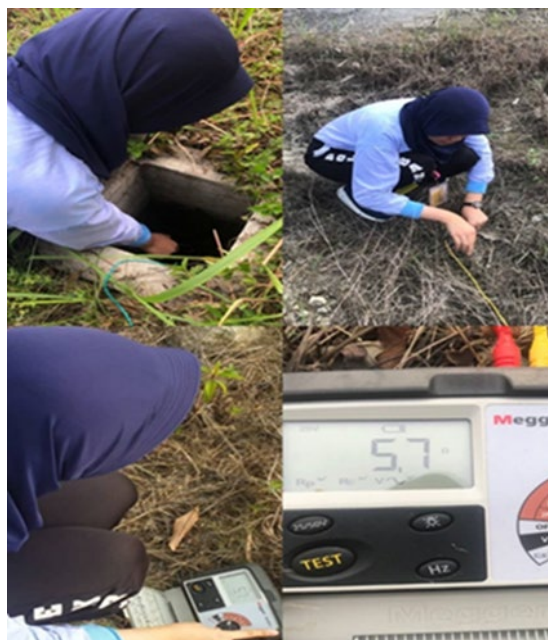
Figure 2. Lightning Arresting Grounding System Measurement
