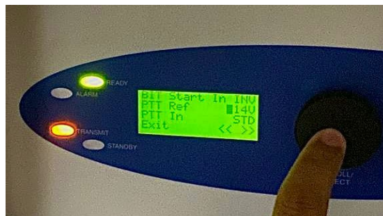
Figure 3. Voltage 14 Volt jumping condition
